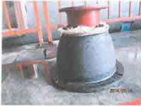
Visual inspection after testing
